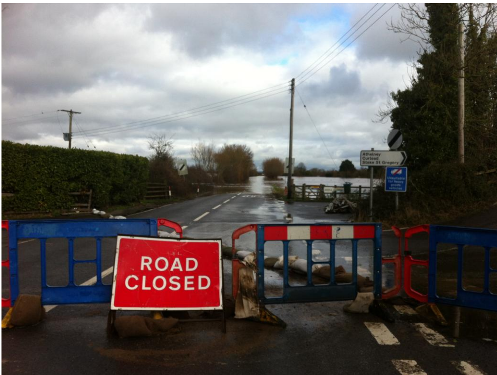
Figure 1: on the road to nowhere. The A361 in the flood area was inundated to the depth of ten feet or more in some places.
